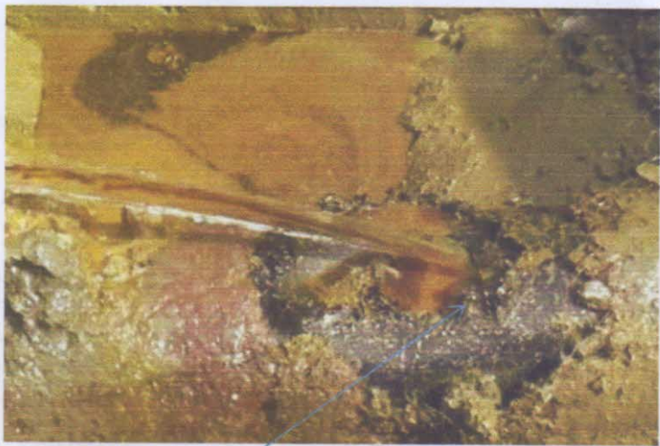
200mm Hacksaw cut on the facility at Point A (Before repair)
