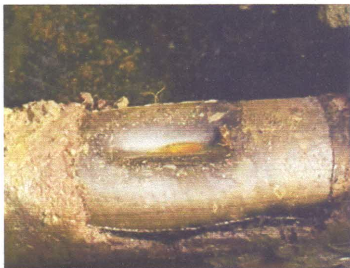
A Section of the Facility, Point B on which Explosive device was used by the Suspect (Before repair)
